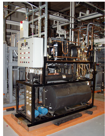
Custom open-frame system is one of several delivering low-temperature water to Cardiac Surgical Suite.
