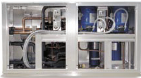
Low-profile, dual-circuit weatherproof chillers are used at a major military contractor facility.
