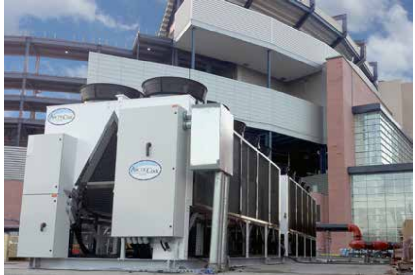
Quietly Keeping Sports Fans Cool Arctic Cool was chosen to provide their remarkable air cooled chillers with highest energy efficiency, lowest noise-levels and integrated free-cooling.
